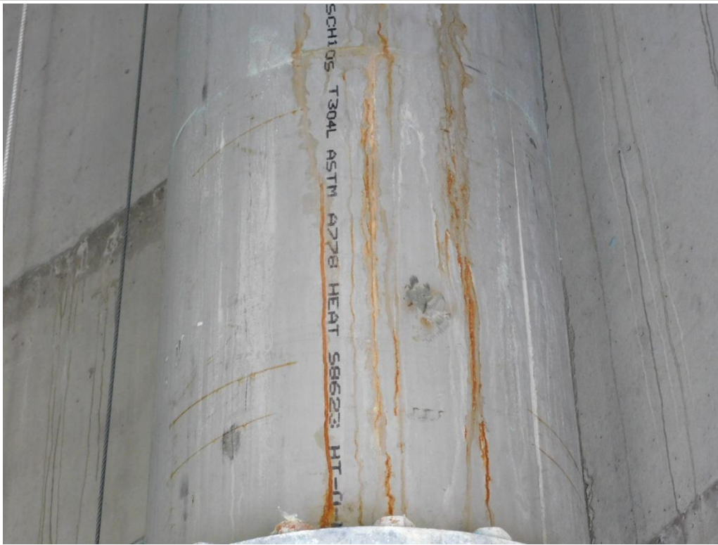
Photograph #: 3 Date: September 2, 2025 Subject: Inlet/Outlet Pipe Designation – SCH10S T403L
