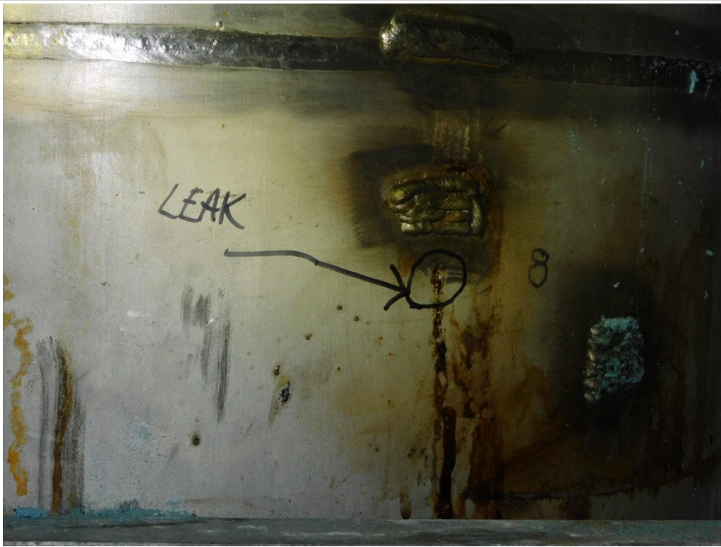
Photograph #: 9 Date: September 2, 2025 Subject: Weeping Water Leak (~24 feet)
