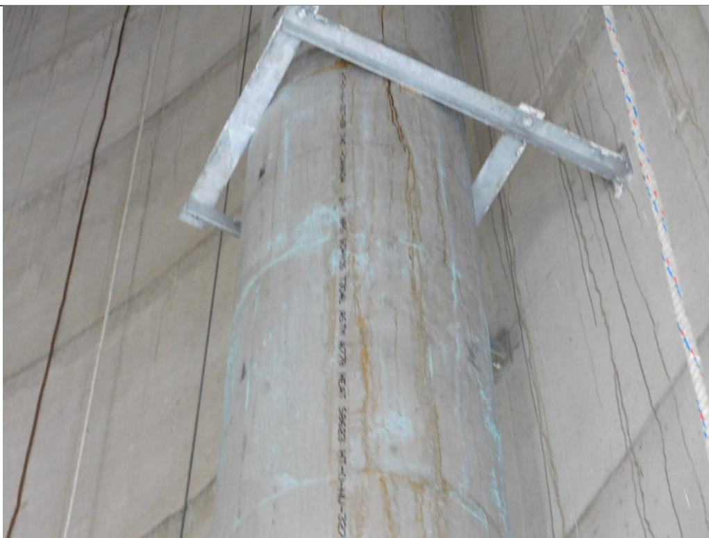
Photograph #: 12 Date: September 2, 2025 Subject: Rust Staining Identifying Additional Potential Leak Locations (Not Active)
