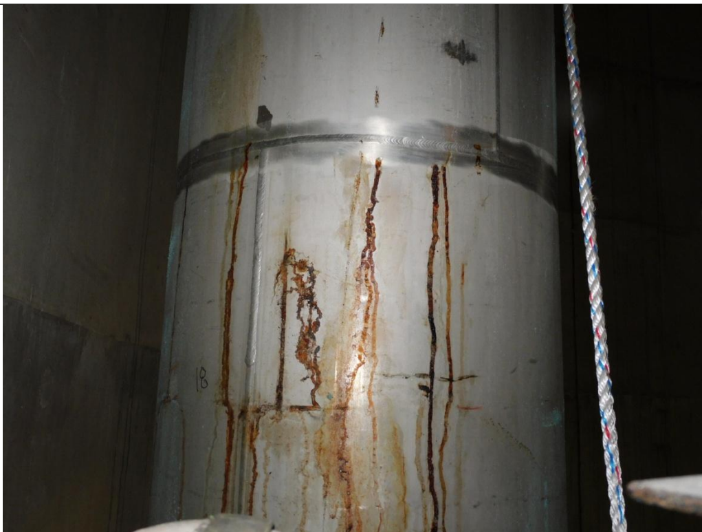
Photograph #: 8 Date: September 2, 2025 Subject: Inlet/Outlet Pipe Rust Staining (Typical)
