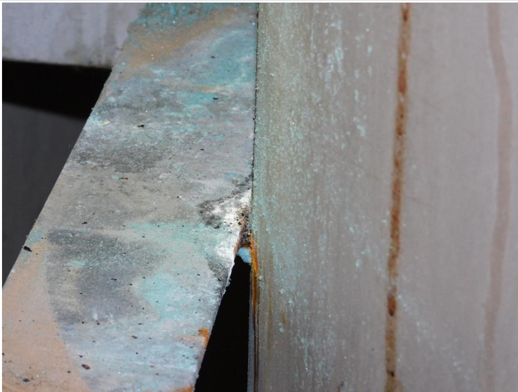
Photograph #: 5 Date: September 2, 2025 Subject: Inlet/Outlet Pipe and Support Dissimilar Metals Contact
