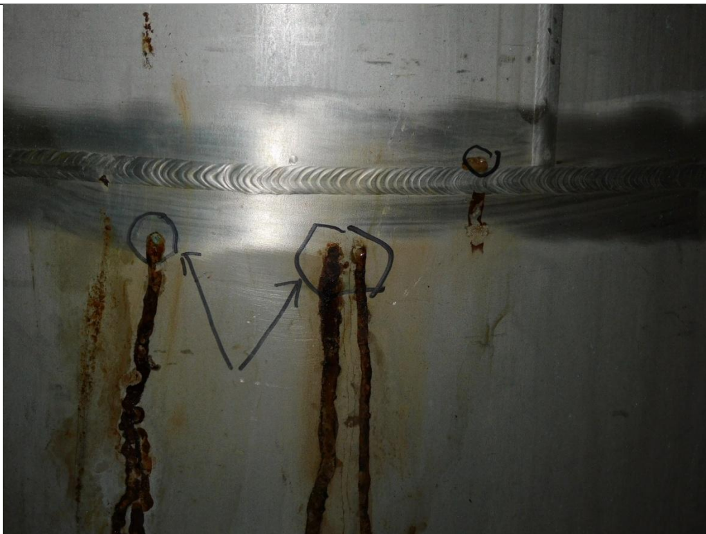
Photograph #: 10 Date: September 2, 2025 Subject: Weeping Water Leaks (~54 feet)
