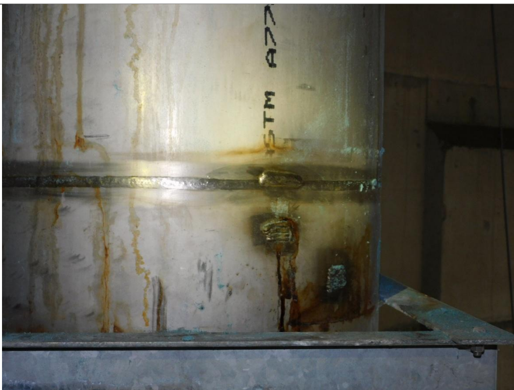
Photograph #: 6 Date: September 2, 2025 Subject: Previous Inlet/Outlet Pipe Repair Welds ('24 feet)
