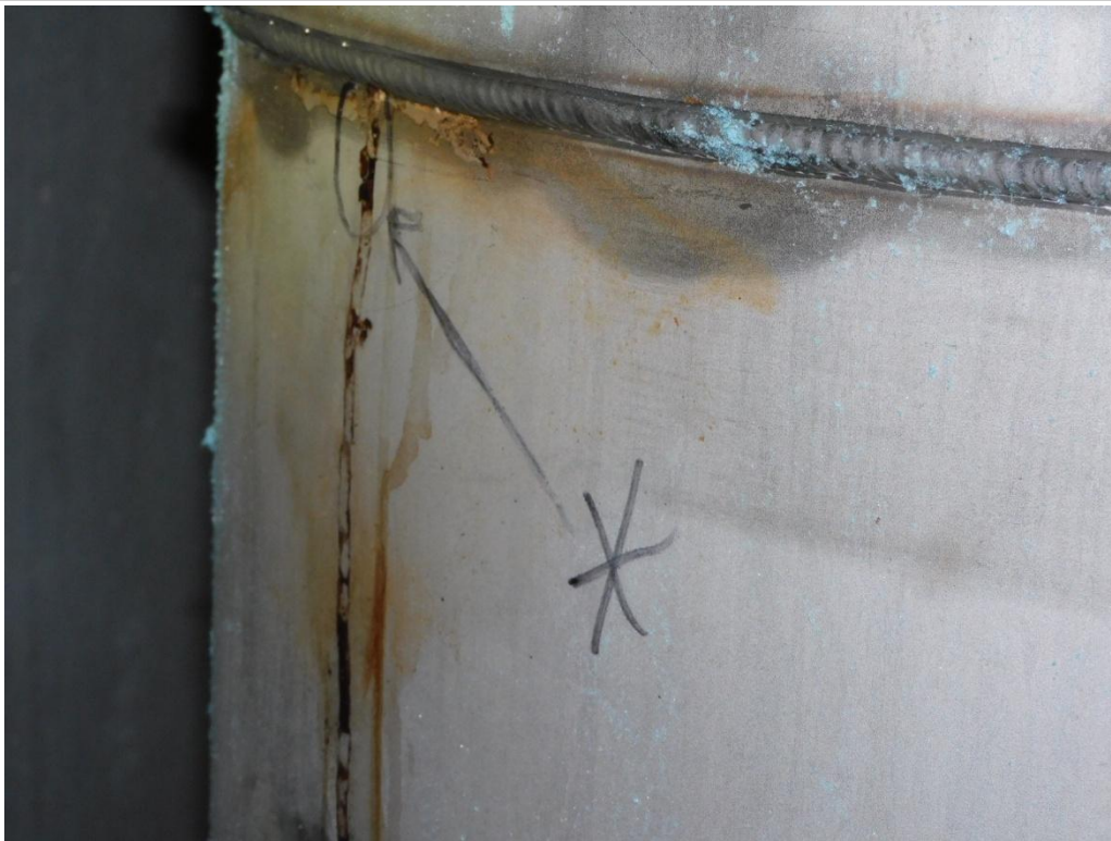
Photograph #: 11 Date: September 2, 2025 Subject: Active Leak with Fine Spray (~60 feet)
