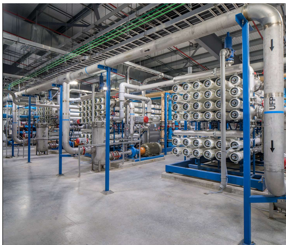
Figure 2-9. Example Membrane Facility (1)
