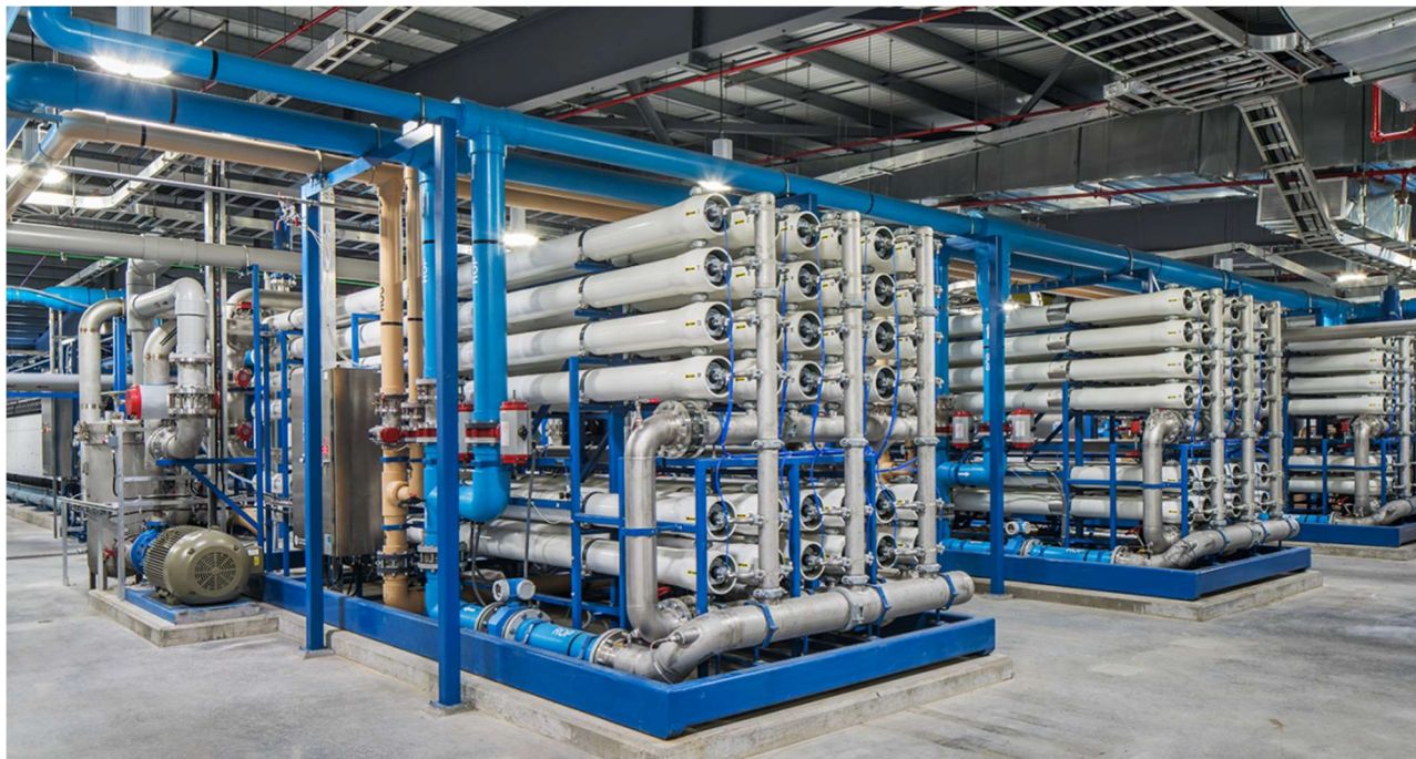
Figure 2-10. Example Membrane Facility (2)
